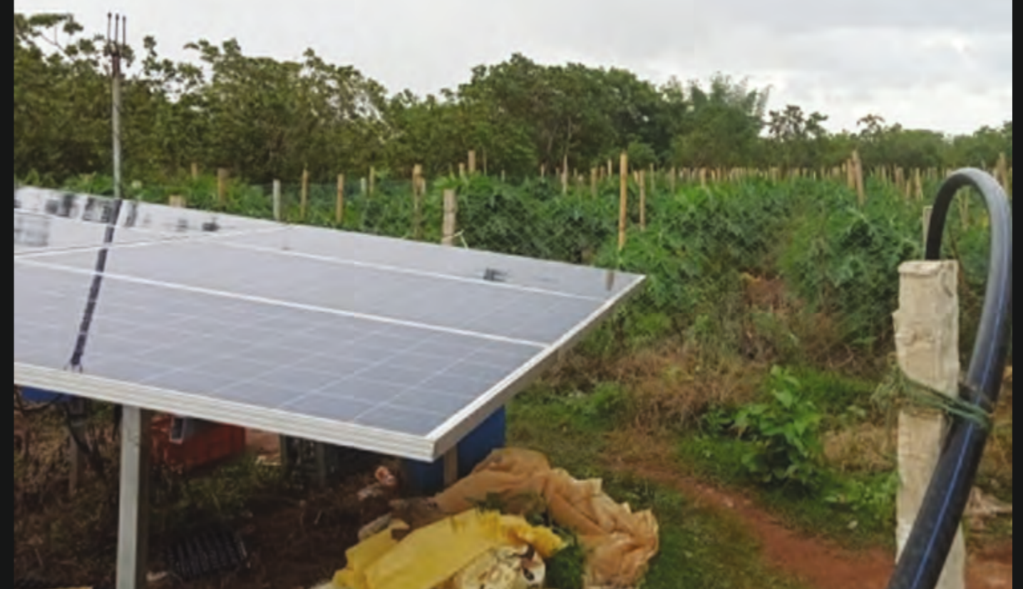
Solar Borewell installed at Salamundali village, Udala Block of Mayurbhanj
