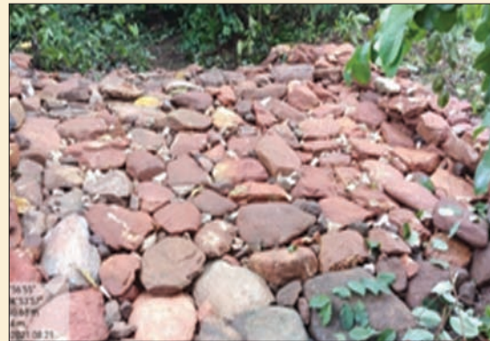
Loose Boulder Check Dam Banki Range, Sundargarh
