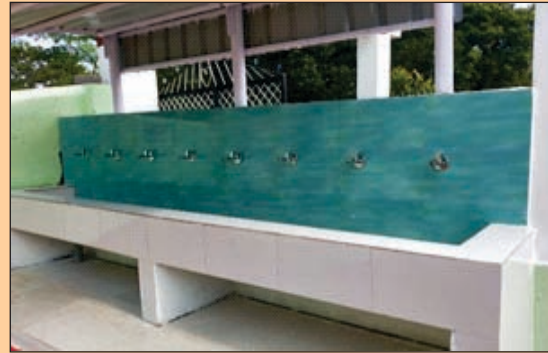
Drinking water facility
