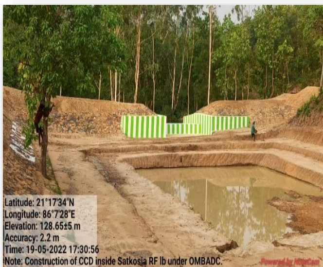
Checkdam at Satkosia , Mayurbhanj
