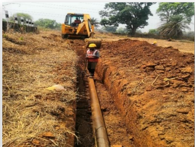
Laying of Pipelines in Mega PWS to Lephripada, Tangarapalli, Sundargarh, Subdega & Balisankara etc.
