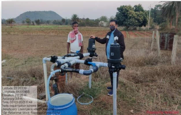
Drip irrigation system installed in Sundargarh
