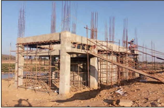
Intake well of Mega PWS of Kutra, Sundargarh District
