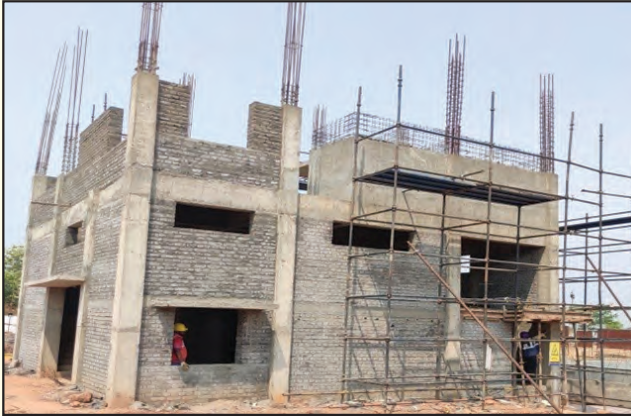
Chemical House at WTP of Mega PWS of Rairangpur, Mayurbhanj
