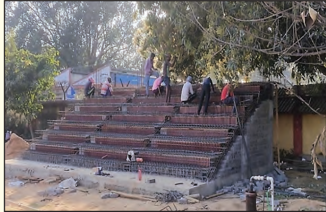
Development of Playground (Construction of Gallery under Progress) at UGIE- Rourkela, Sundargarh
