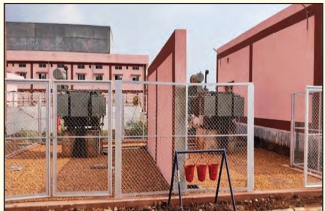
WTP site at Belda, Mega PWS to 115 mining affected villages of Keonjhar
