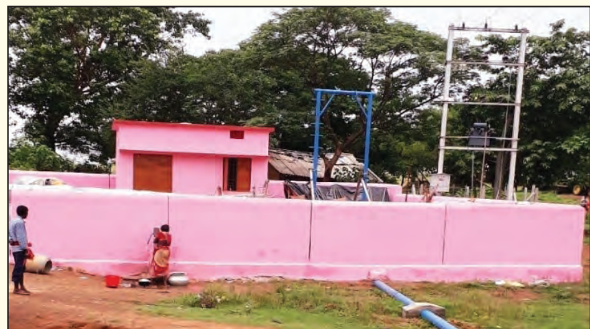
Pump House at Vyasagar ULB, Jajpur District
